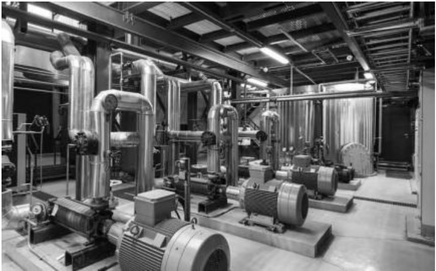
Figure 69. Pumps in a Power Plant
