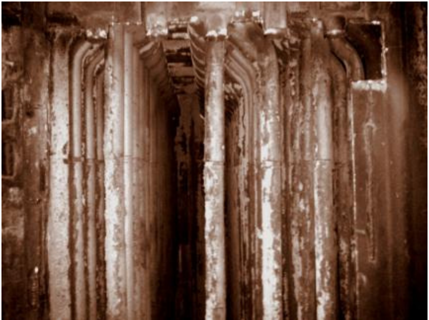
Figure 85. Typical HRSG Superheater Tubes Showing Ageing
