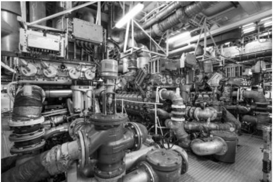
Figure 68. Pipes and Valves in a Power Plant
